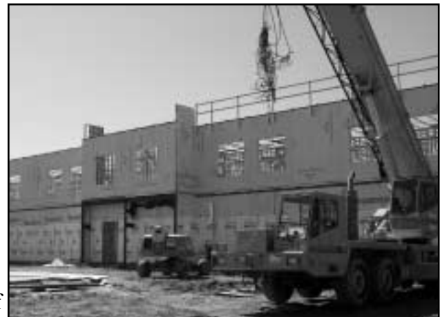
At Newark Charter School's new custom facility, shown here, construction is well underway.
